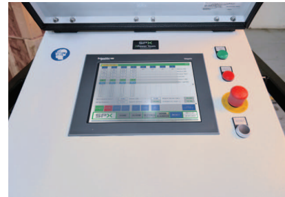
The home screen on the Motion Control System is easy to use and operate. It highlights all activities during use of the Motion Control System. For each cylinder in operation, the cylinders performance is captured and displayed on the HMI screen as illustrated below.
